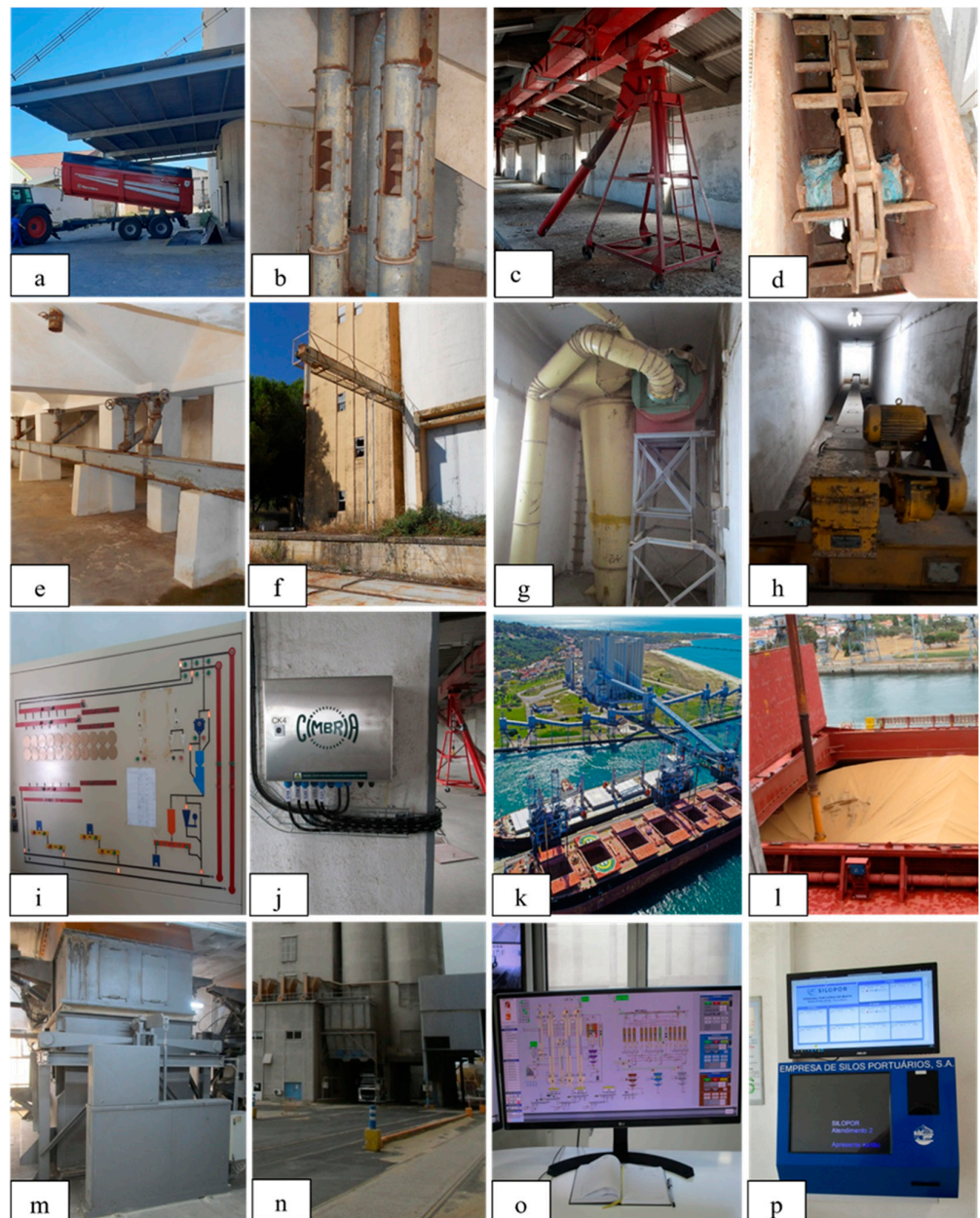
Figure 7. (a) Reception hopper in silo in Aljustrel, Alentejo; (b) grain elevator and detail of elevator scoop in silo in Vila de Boím, Alentejo; (c) upper horizontal belt conveyor and loading tubes in silo in Pavia, Alentejo; (d) detail of drive chain and crossbars inside upper horizontal belt conveyor in silo in Mogadouro, North; (e) offloading tubes and lower horizontal belt conveyor in silo in Mértola, Alentejo; (f) external bulk offloading tube in silo in Portalegre, Alentejo; (g) dust collector in silo in Vale de Figueira, Centre; (h) underground horizontal conveyor from hopper to elevators in silo in Cuba, Alentejo; (i) control panel in silo in Ferreira do Alentejo, Alentejo; (j) temperature sensor controls in silo at Vale de Figueira, Centre; (k) aerial view of Trafaria silos, Lisbon; (l) detail of pneumatic unloader working in Trafaria silos, Lisbon; (m) online scale in Trafaria silos, Lisbon; (n) dispatch cells at Beato silos, Lisbon; (o) computerized control room in silo in Leixões, North; (p) computer terminal for haulers in Beato silos, Lisbon.
