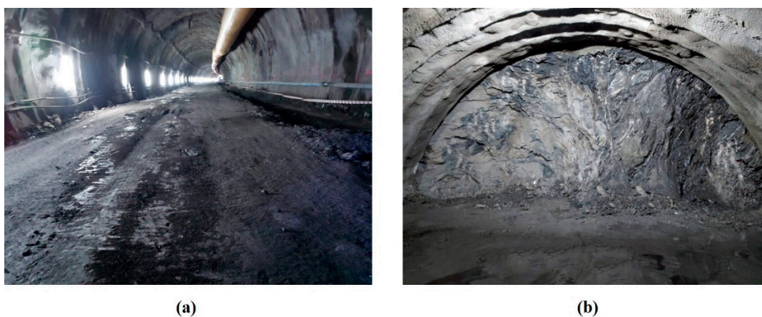
Figure 7. Railway tunnel excavated using the top-heading-and-benching method: (a) full face and forced duct, and (b) top heading.
