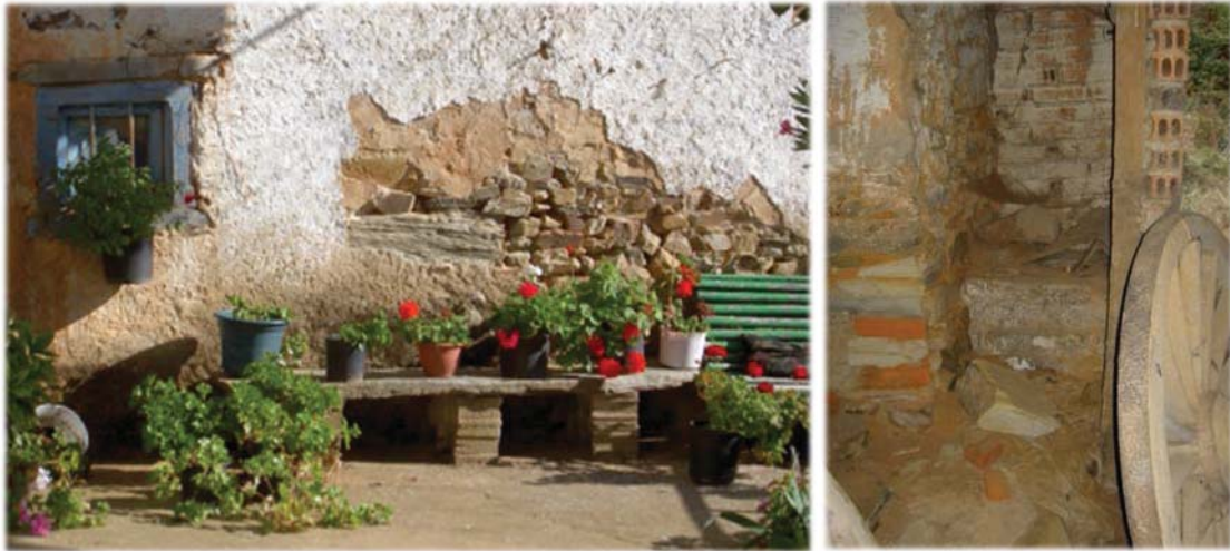
Image 94. Changes in the houses of the lower classes. People who could not afford to build new modern houses started to add toilets (on the right) and new functional areas and materials to the houses when they could afford it. Also, they covered with concrete or limestone the stone walls of their houses, that became a symbol of poverty. Source: Author.
