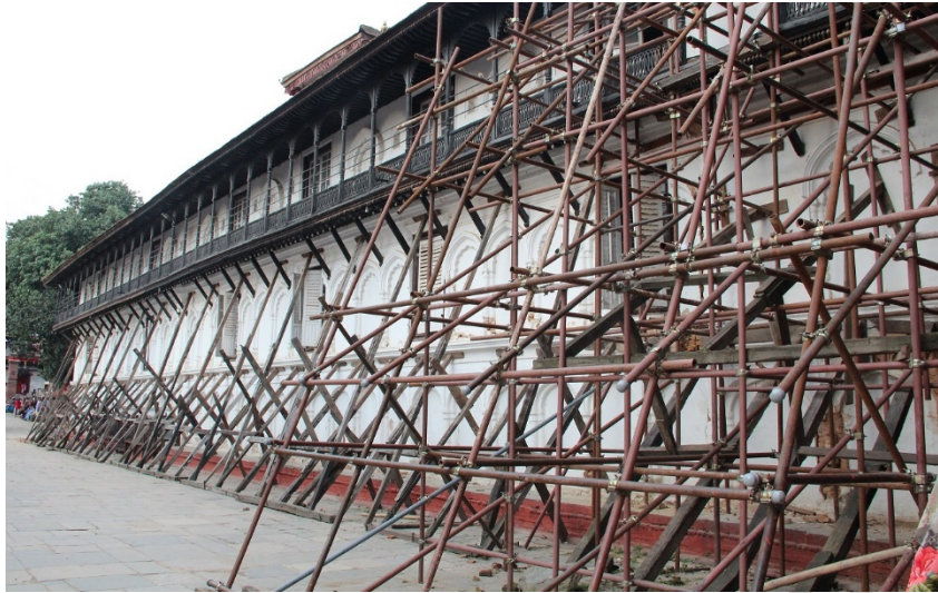
Figure 10: Earthquake damaged heritage building in Nepal supported by poles and scaffolding.
