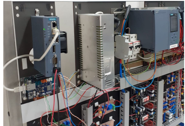
Figure 4: Physical appearance of the IOT 2050 installed in the smart microgrid.
