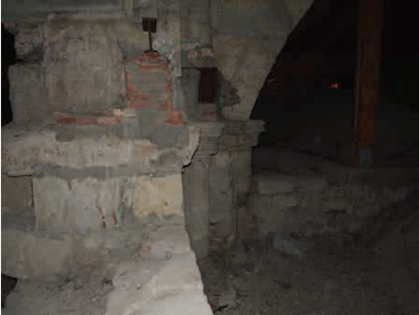
Fig. 10. Palencia Cathedral. Pillar over the ceiling in the epistle aisle. Photo by the author.
