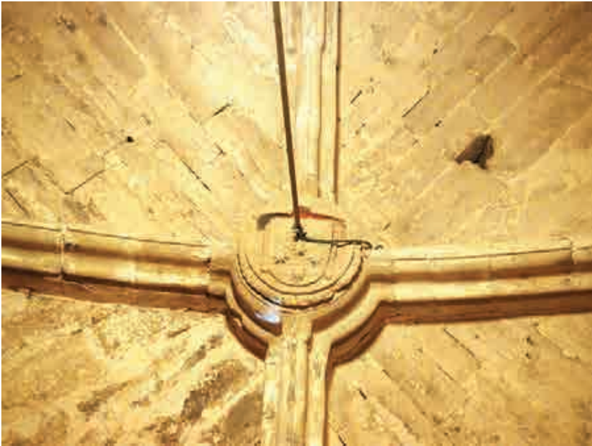
Fig. 7. Palencia Cathedral. Vault on the lower part of the tower. Photo by the author.
